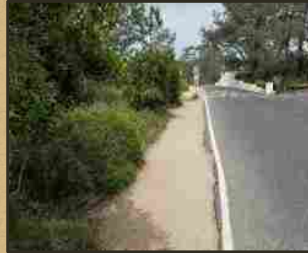
Non-compliant trails and walkways
