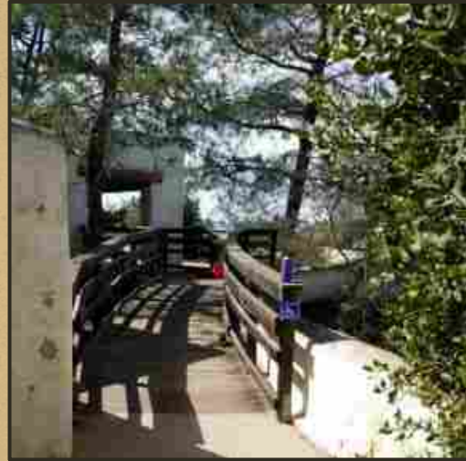
Ramp is non-compliant and not to current code
