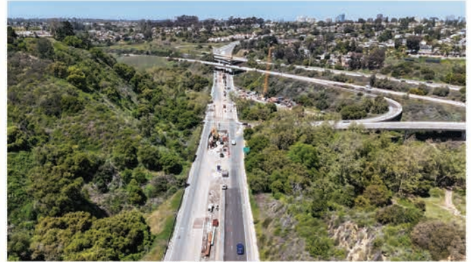
Above: Tunnel construction is now ongoing in the center of Genesee Avenue and in the Marian Bear Park Genesee Avenue parking lot.
